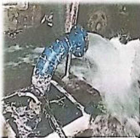
Test run @50 Hz VFD setting with stable discharge of Q = 36 LPS
